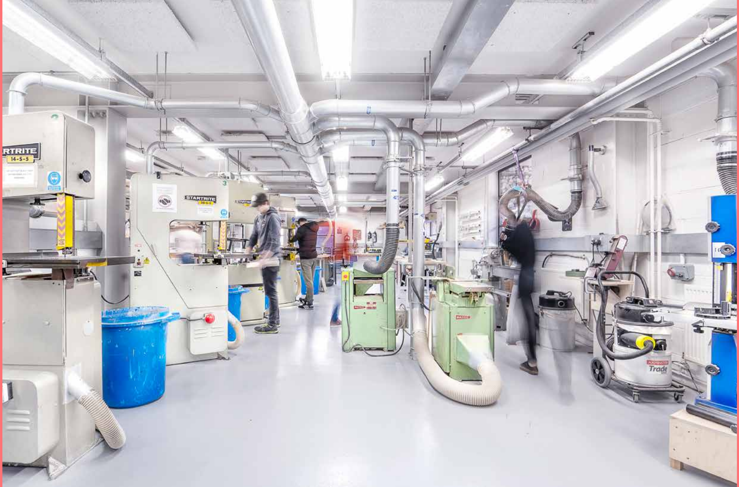
+ Our purpose built workshop is fitted with industry-standard equipment.
